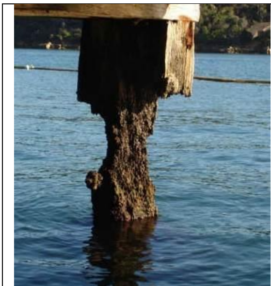
Pile in very poor condition
