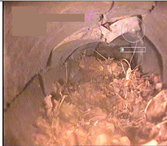
Pipe in very poor condition
