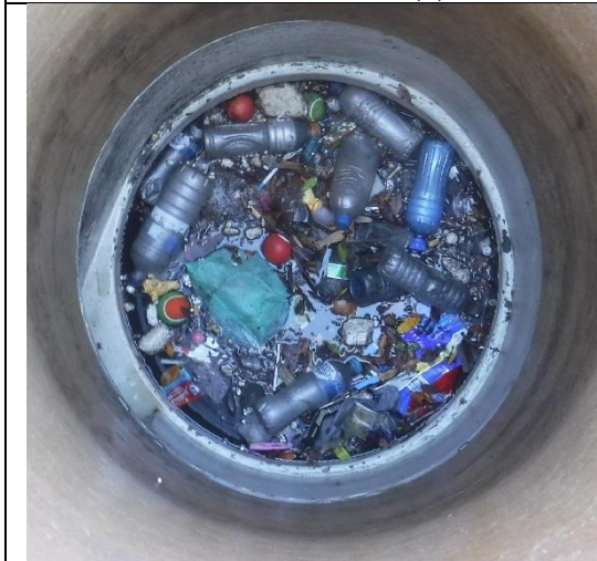
Gross Pollutant Trap prior to cleaning
