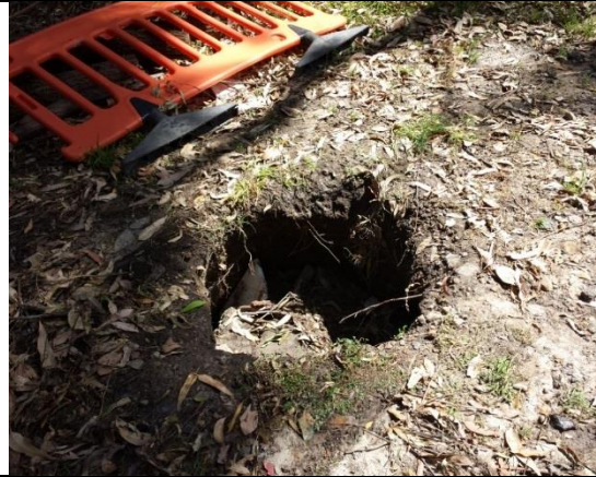
Sink hole in reserve near pipe
