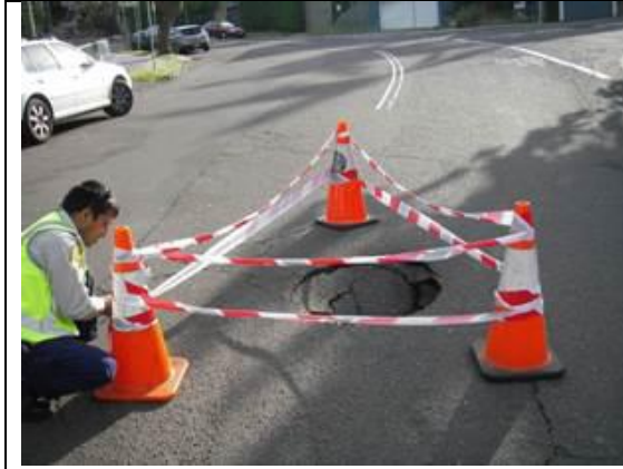
Sink hole in road near pipe
