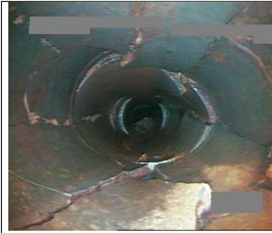
Pipe in very poor condition
