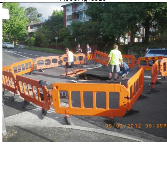
Sink hole in road near pipe
