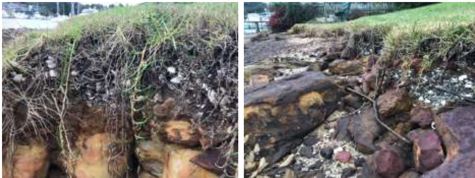
Coastal erosion monitoring, Bayview
