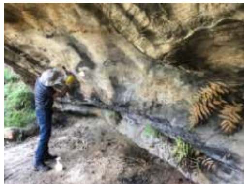
Graffiti removal, North Wahroonga
