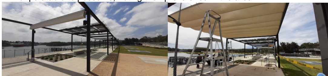
Photographs of new shade cloth provided by North Sydney Council
