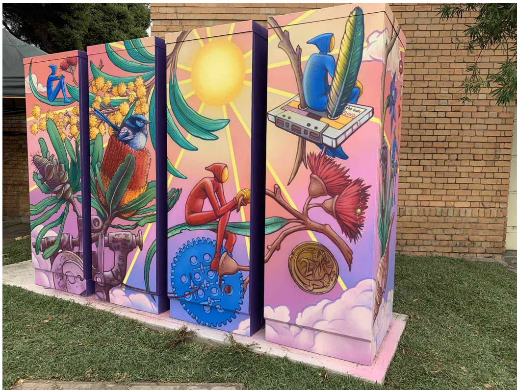
Fig 3. City of Yarra community battery
