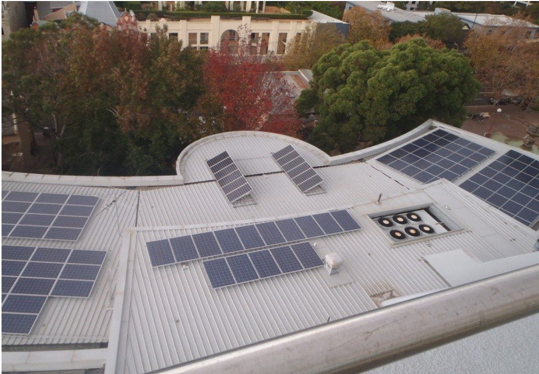
Solar Panels have been rolled out across a number of Councils Community and operational buildings over the last 5 years as part of an ongoing program. Stanton Library
