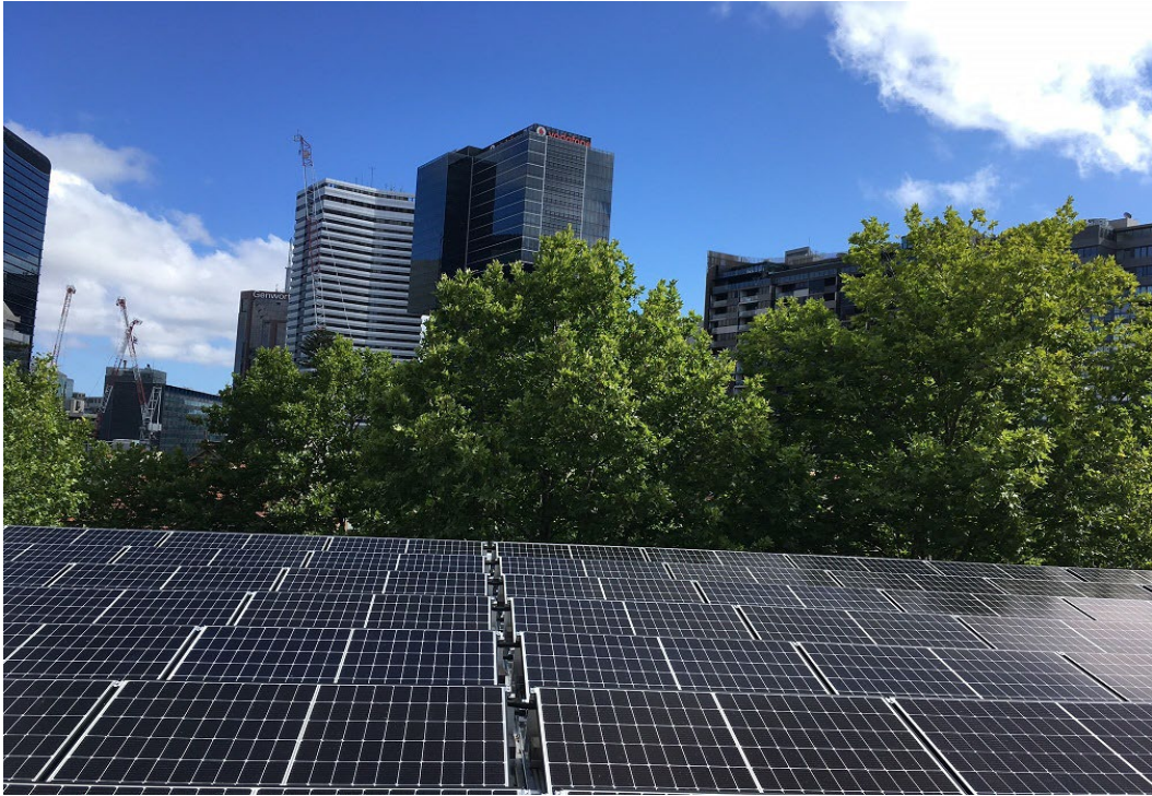
Solar Panels have been rolled out across a number of Councils Community and operational buildings over the last 5 years as part of an ongoing program. North Sydney Council Chambers Wyllie Wing roof
