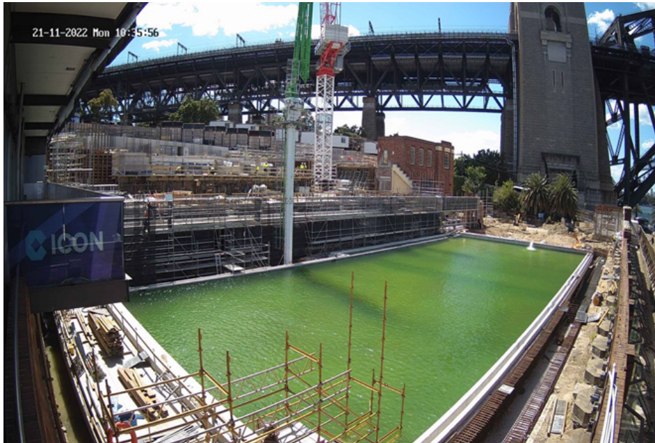
50m pool ready to water test 21/11/2022 - Major Milestone with the 50m pool filled with water for the first time.
