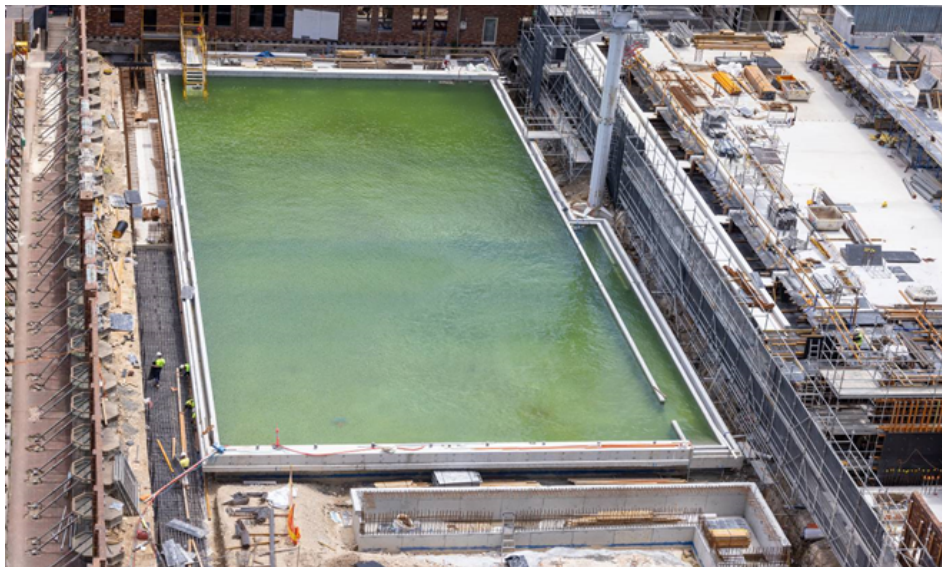
50m pool ready to water test 21/11/2022 - Major Milestone with the 50m pool filled with water for the first time.
