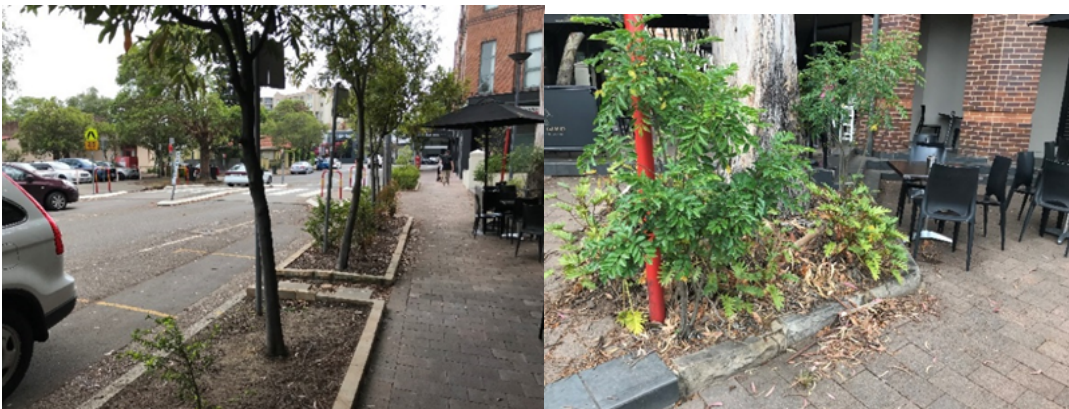
Photos 9-10 Langley Place – unkept planter beds – old paving that is at the end of its useful life
