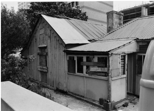
Figure 2. 38: View of the north elevation of the house and entry porch leading into the rear kitchen wing of Don Bank prior to restoration. Source: Stanton Library
