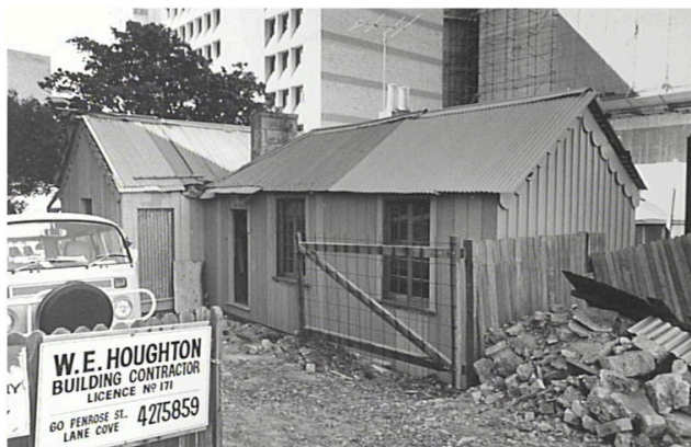
Figure 2.46: The rear wing of Don Bank during restoration works c.1980. Source: Stanton Library (PF 2420)
