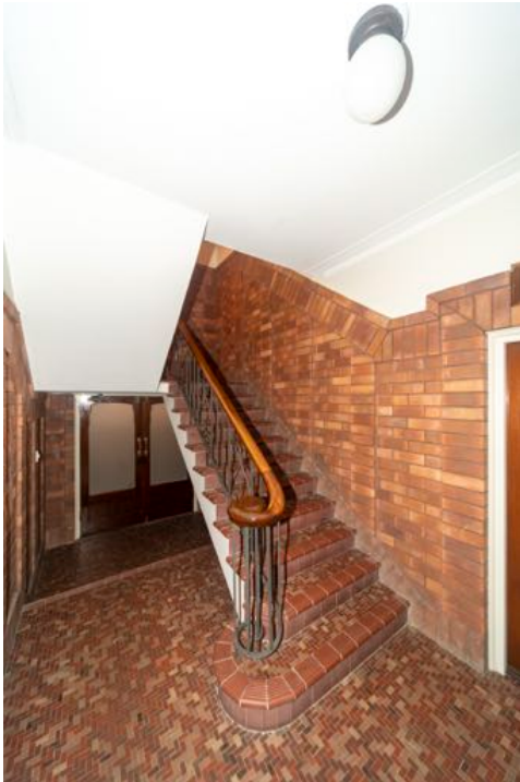
Figure 16: (Left) Original stairway in lobby showing original staircase, original tiling and brick and plaster wall finish
