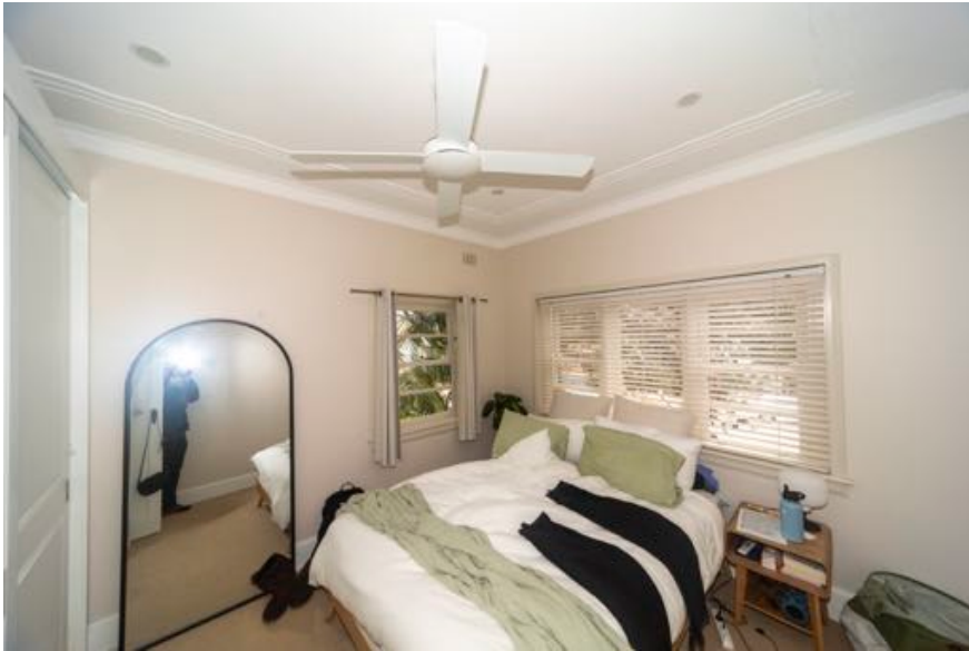
Figure 32: Unit 1 bedroom with original ceiling
