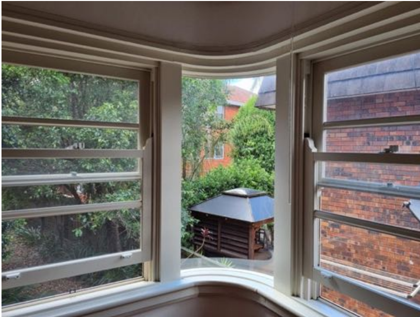
Figure 24: Curved glass to corner, with typical timber framed double hung windows with horizontal glazing bars to either side. Source: photo supplied by North Sydney Council
