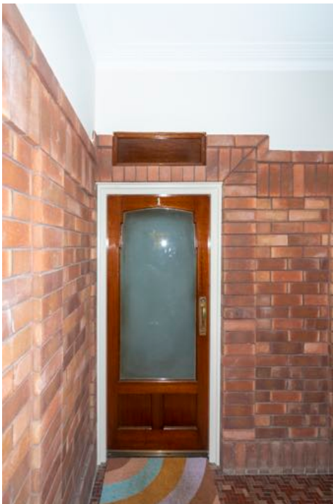
Figure 17: (Left) Unit 1 internal entry door
