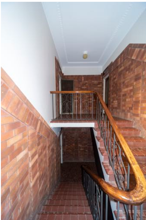
Figure 23: (Left) View of stairway to 1 st floor lobby, noting original 1 st floor lobby ceiling, brickwork, plasterwork, tiling and original stairway details.
