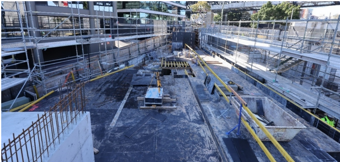
Level 4 NW plant room 27/7/2023
