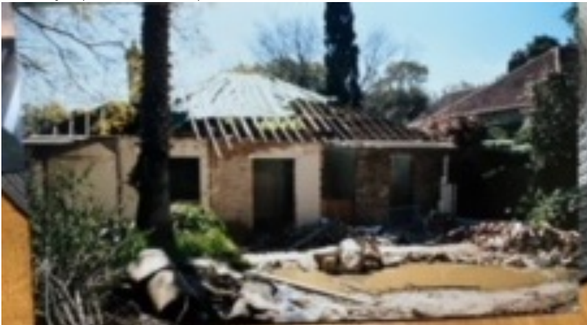
1998 photo of the house at 7 Selwyn Street during construction of 1997-1998 alterations and additions. Source: Photo shown by the property owner, image of photo taken on mobile phone at the site.
