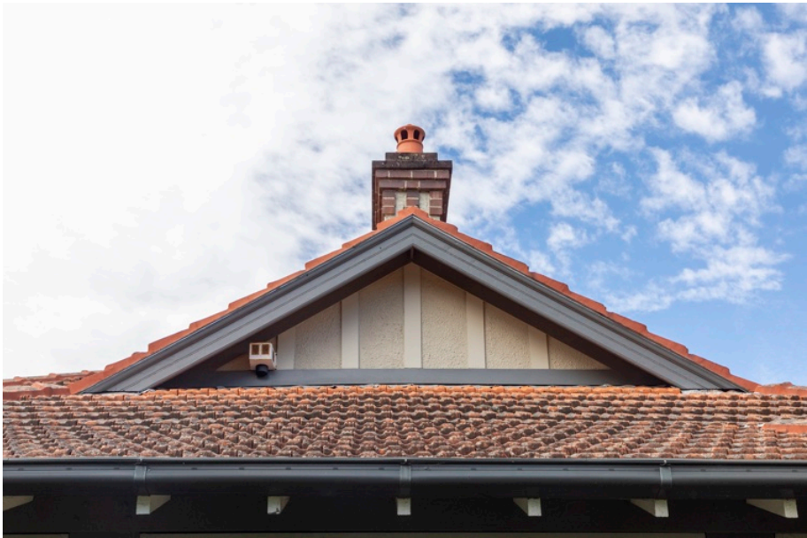
Figure 20: Roof detail. Chimneys were reconstructed as part of the 1997 work to the house.
