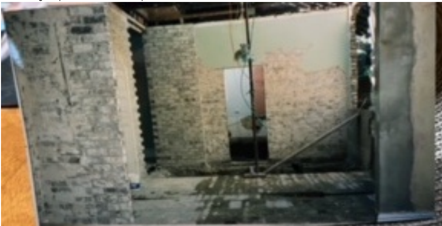
1998 photo of the house at 7 Selwyn Street during construction of 1997-1998 alterations and additions. Source: Photo shown by the property owner, image of photo taken on mobile phone at the site.
