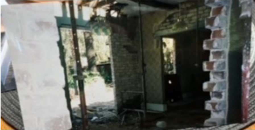
1998 photo of the house at 7 Selwyn Street during construction of 1997-1998 alterations and additions. Source: Photo shown by the property owner, image of photo taken on mobile phone at the site.
