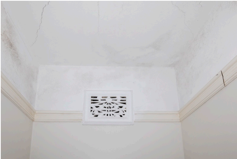
Figure 74: Detail of plaster vent and picture rail above the cupboard in the same room. Note cracking to ceiling above the cupboard indicates this may be a small original section of plaster ceiling.
