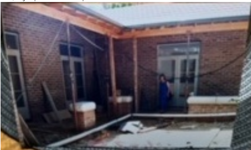
1998 photo of the rear of the house at 7 Selwyn Street during construction of 1997-1998 alterations and additions. Source: Photo shown by the property owner, image of photo taken on mobile phone at the site.
