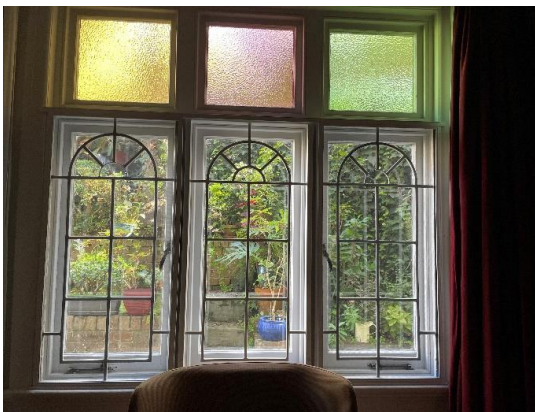
Figure 5.35 First floor apartment to west— original timber-framed casement windows with stained glass.
