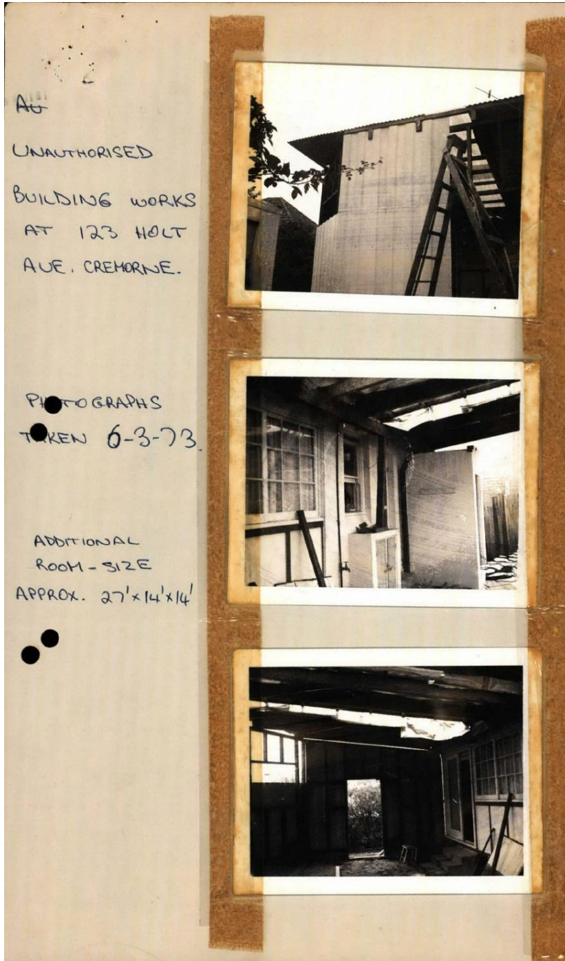
Figure 4.4 Three views showing unauthorised building works, 123 Holt Avenue, 6 March 1973. (Source: North Sydney Council, P339/123/3)
