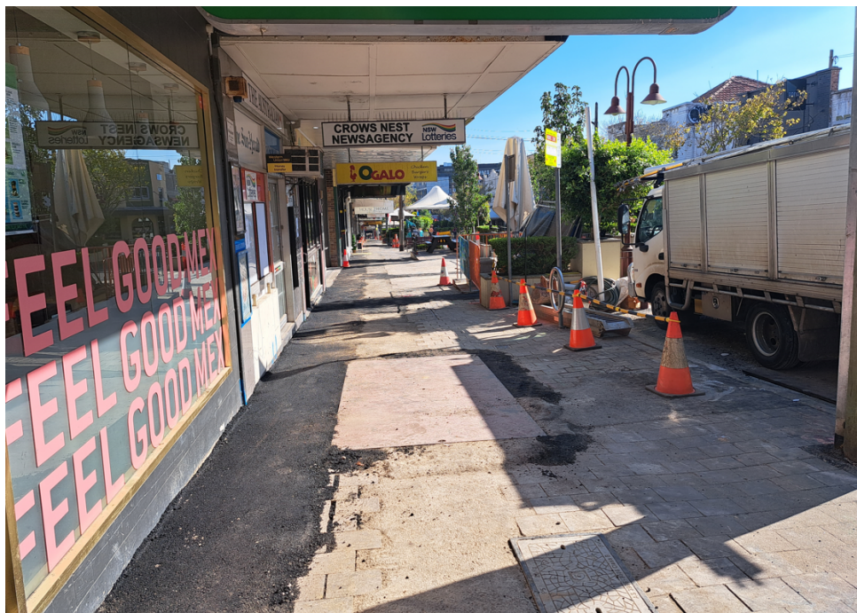
Photo 1 Willoughby Road (West side) showing uneven footpath disturbed by service trenches
