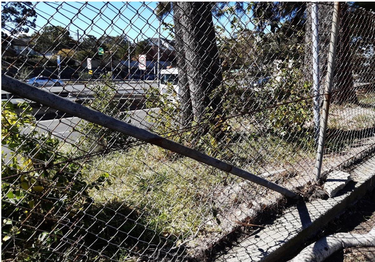
Photo 11 - Proposed Location of RMS noise wall at North Eastern end of Jenkins Lane adjacent to Warringah Freeway
