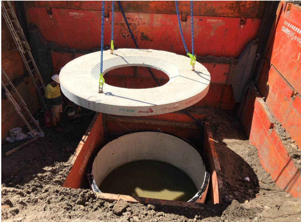
Image of what the Hayes Street GPT will look like - New GPT being installed (Little Young Street 2018)
