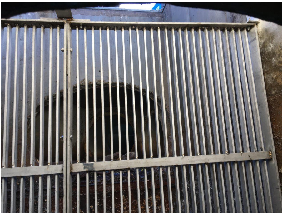
New trash racks (installed 2017)
