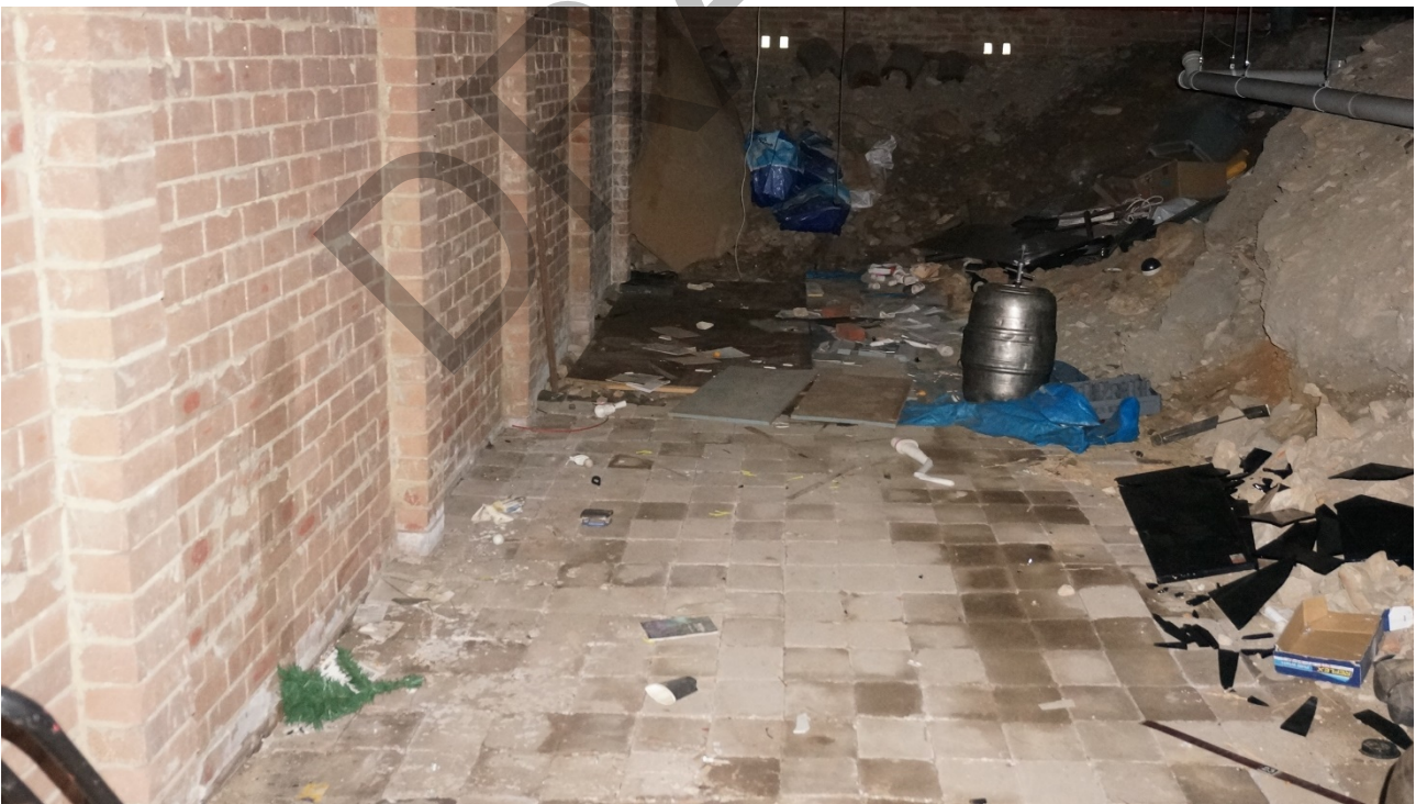
12. View across sub-floor area to the west. The area had been used for storage purposes. High voltage equipment was not present in the area contrary to the high voltage warning sign on the access door. Sandstone rubble fill, visible on the right of the image, appeared to extend below the building.
