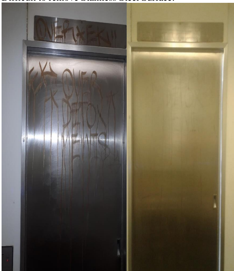
Before and after photos of typical instances of “hard to remove graffiti” in North Sydney on Council Infrastructure – Etched into Stainless Steel - Exeloo public toilets at Bradfield Park (South), Milsons Point.
