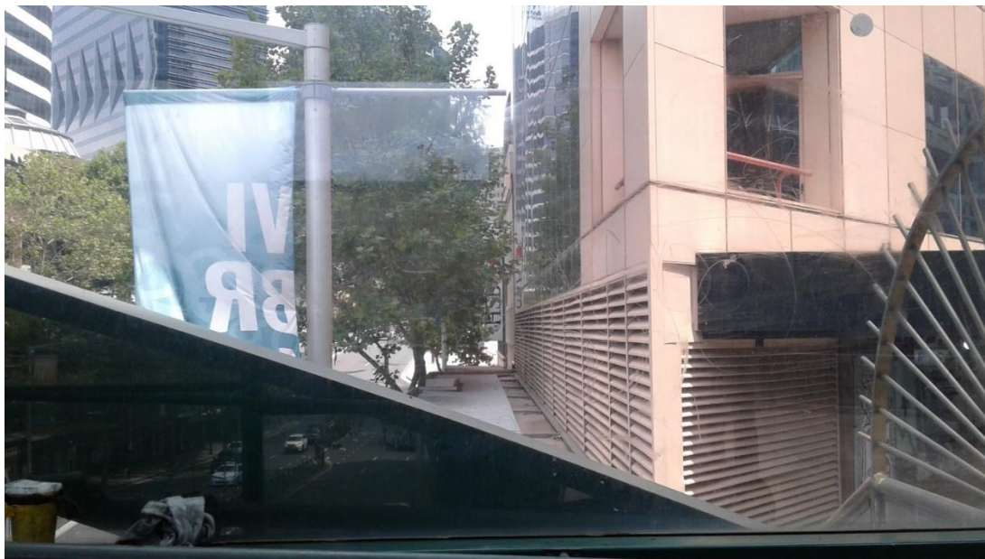
Before and after photos of typical instances of “Glass etching” in North Sydney on Council Infrastructure – Council’s Footbridge over the Pacific Highway – North Sydney Centre. (Note how the etched glass could not be removed completely).
