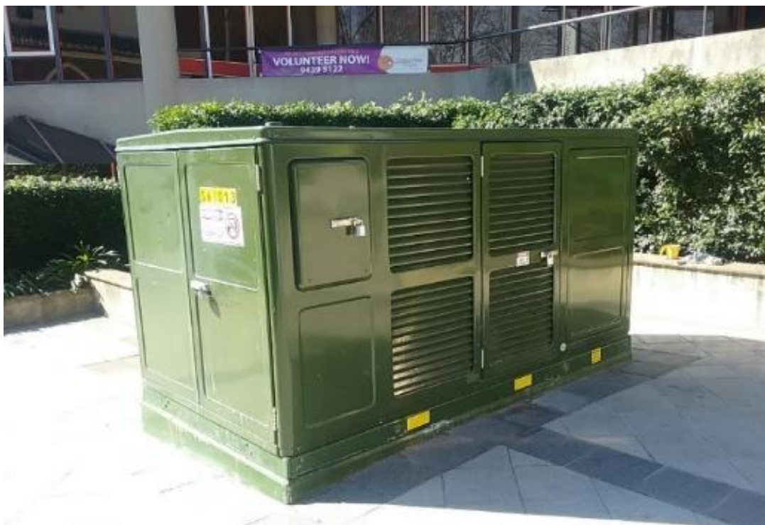
Before and after photos of typical graffiti in North Sydney on Utility Company Infrastructure – North Sydney Council removes graffiti from utility Company Infrastructure “ Free of Charge ” to ensure the visual amenity of Council’s Public domain is always kept to a high standard - Substation Energy Australia at Crows Nest Community Centre.
