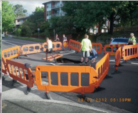
Sink hole in road near pipe
