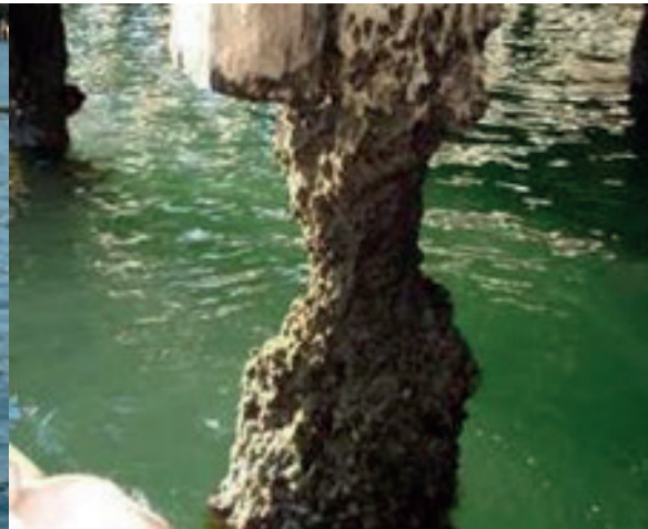
Pile in very poor condition
