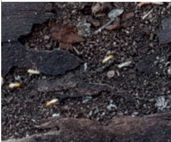
Termites found in timber marine structure
