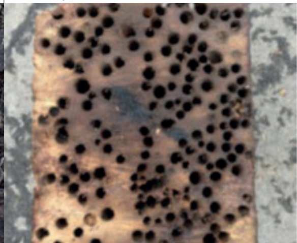
Evidence of marine worms in timber structure
