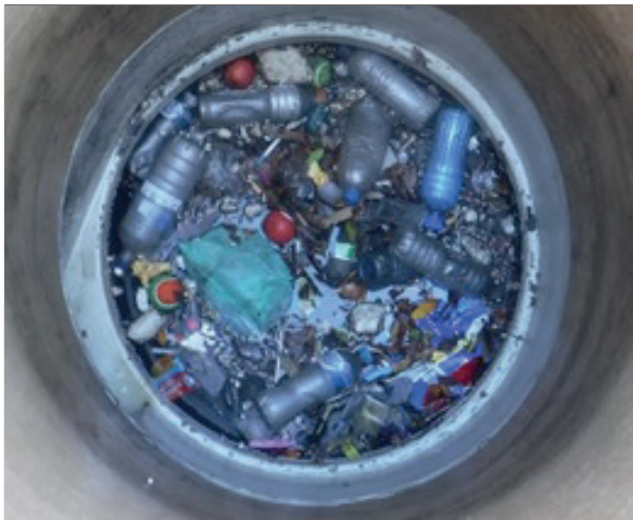
Gross Pollutant Trap prior to cleaning
