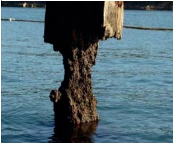
Pile in very poor condition
