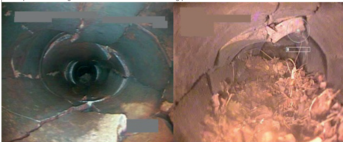
Pipe in very poor condition
