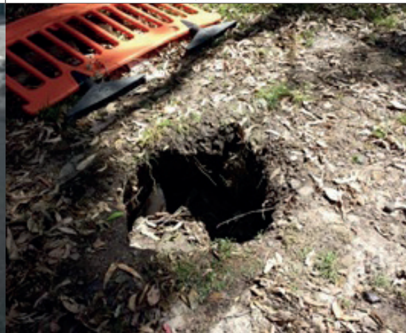
Sink hole in reserve near pipe
