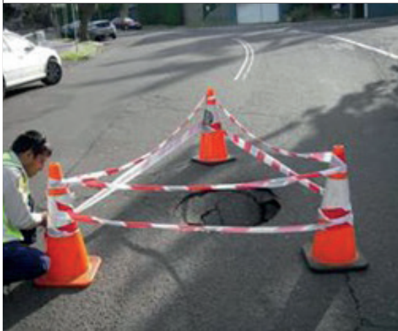
Sink hole in road near pipe
