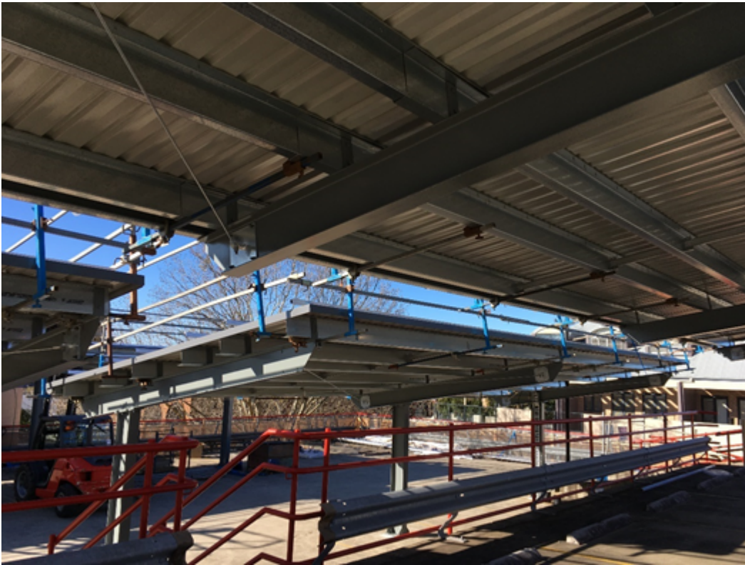
Rails installed for solar PV panels to be mounted on
