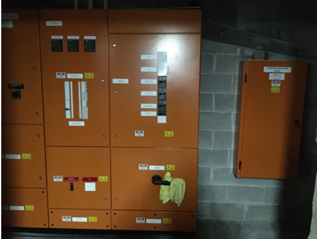
New main switchboard at Holtermann Street Car park
