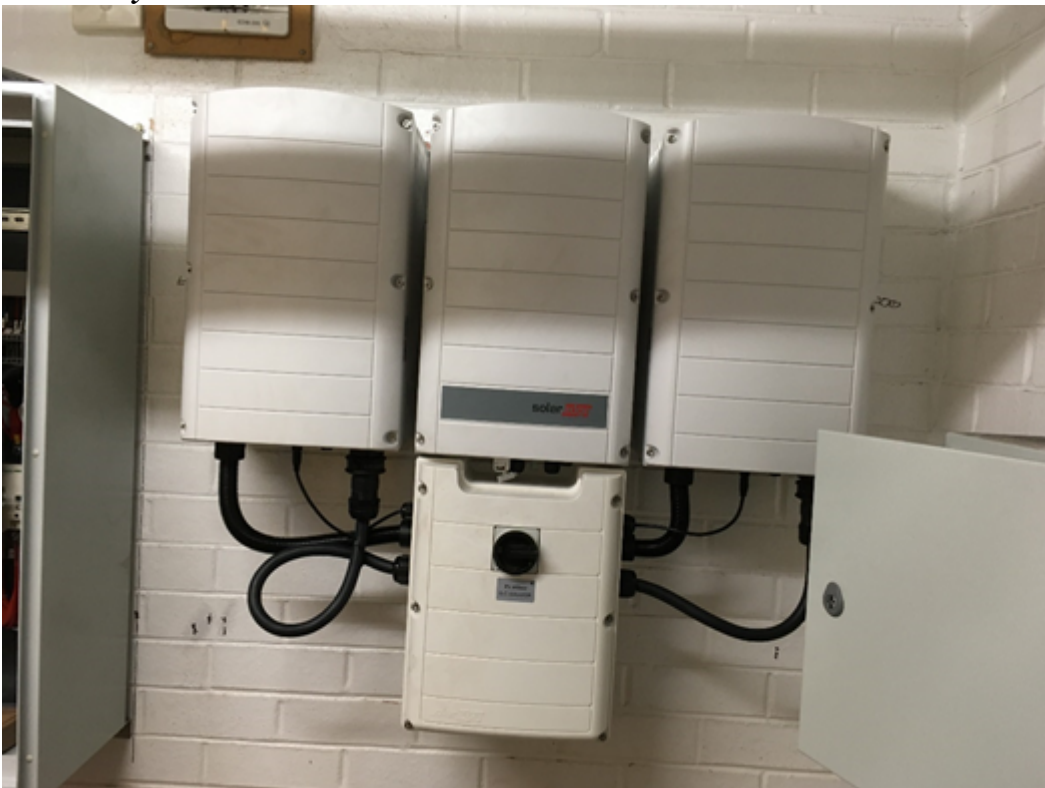
Solar PV system Inverters
