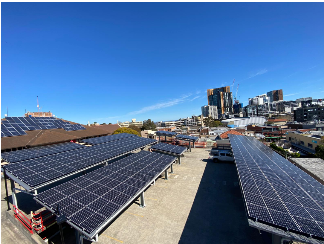
282 x Trina Solar panels at Holtermann Street Car Park roof level
