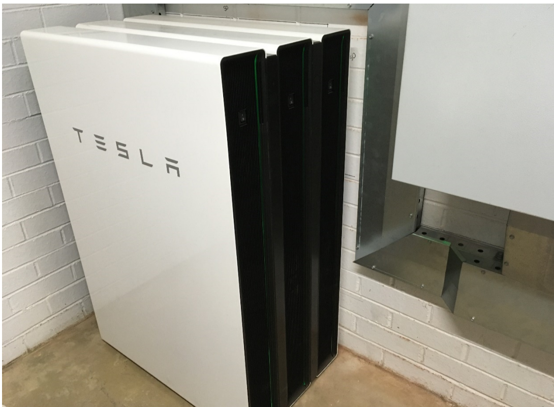
3 x Tesla Powerwall batteries for the Solar PV system
