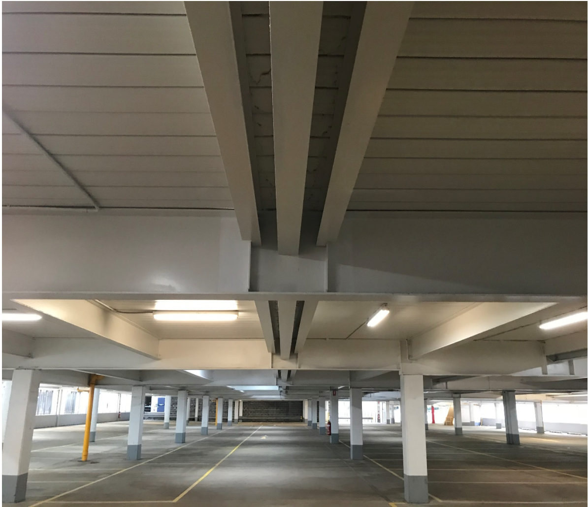
Photo of Ward Street carpark – Structural Repairs and painting undertaken by Wilson parking as part of the handover to Council on 23 August 2020.
