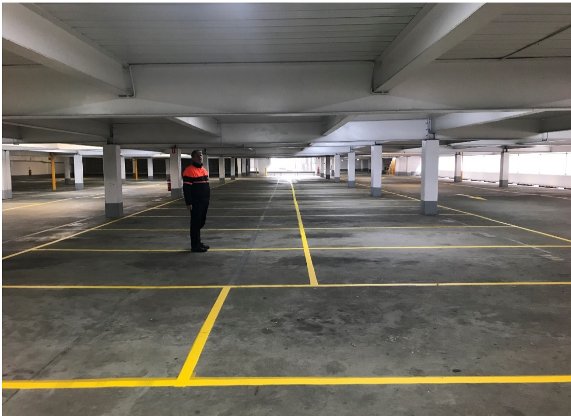
Photo of Ward Street carpark – Level 2 – new line marking undertaken by Wilson parking as part of the handover to Council on 23 August 2020.
