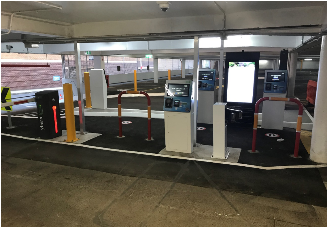
Photo of Ward Street carpark – New Carparking Equipment installed at entry to the carpark by NSC after takeover on 23 August 2020.
