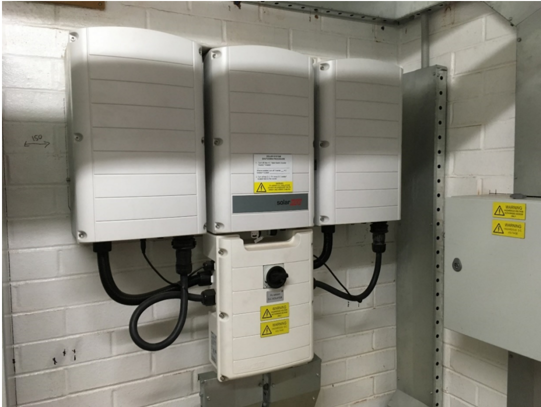
SolarEdge Inverters for the Solar PV system at Holtermann St Car Park
