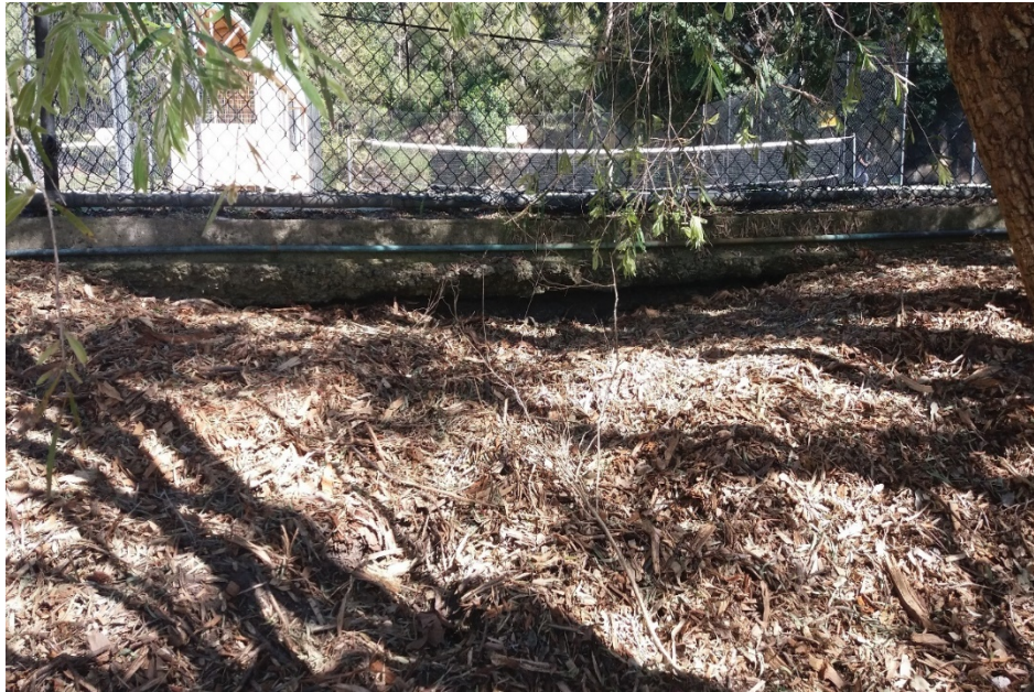
Photo 13 - Primrose Park - flooding 27 November 2018 - 1:100-year storm event - "washout" area under the courts after the November 2018 flooding
