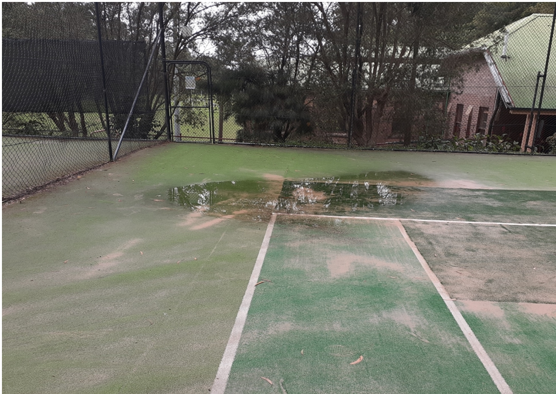
Photo 5 – Existing Primrose Park Tennis Courts – “Ponding” indication subsidence of the courts Photo August 2019
