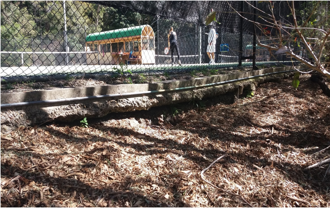
Photo 4 – Existing Primrose Park Tennis Courts – “Washout” under courts Photo August 2019
