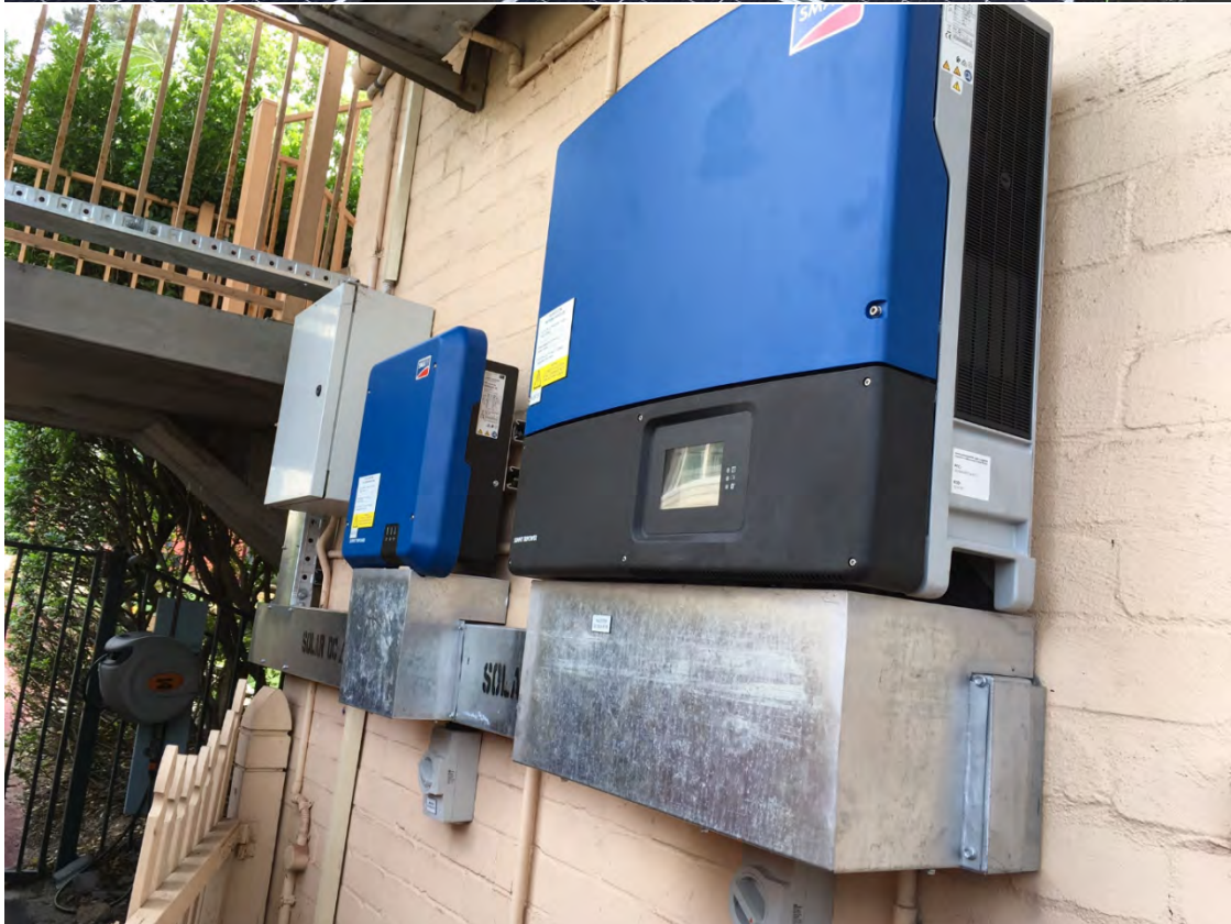
McMahons Point Community Centre new inverters. The total system capacity is 21.5 kW comprising two systems – 6.5 kW for the Community Centre and 15 kW for the
