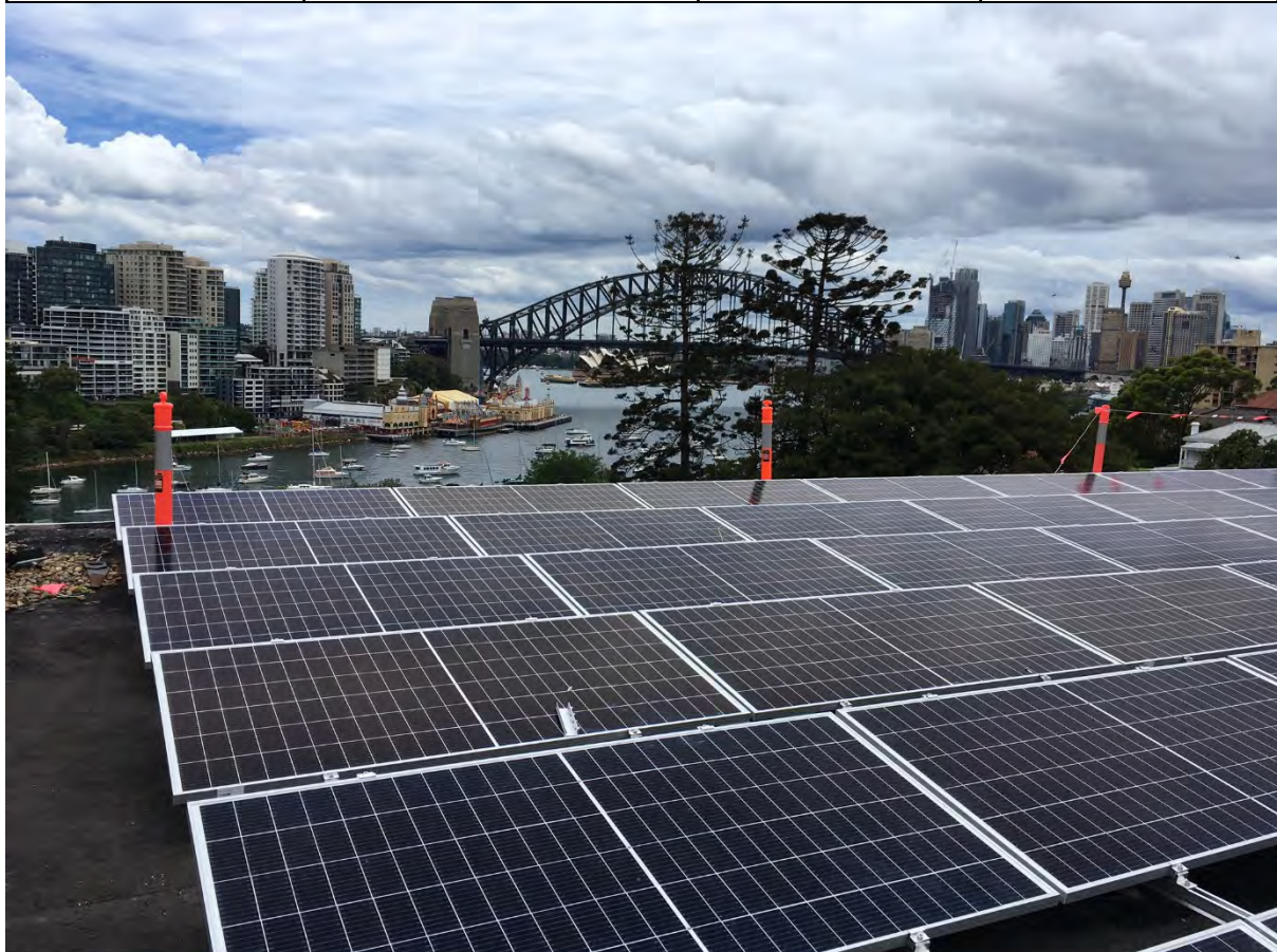
McMahons Point Community Centre new solar panels.
