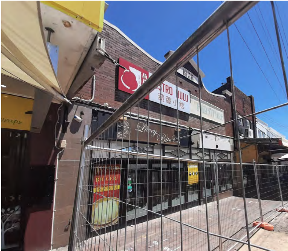
Willoughby Road Façade to be restored
