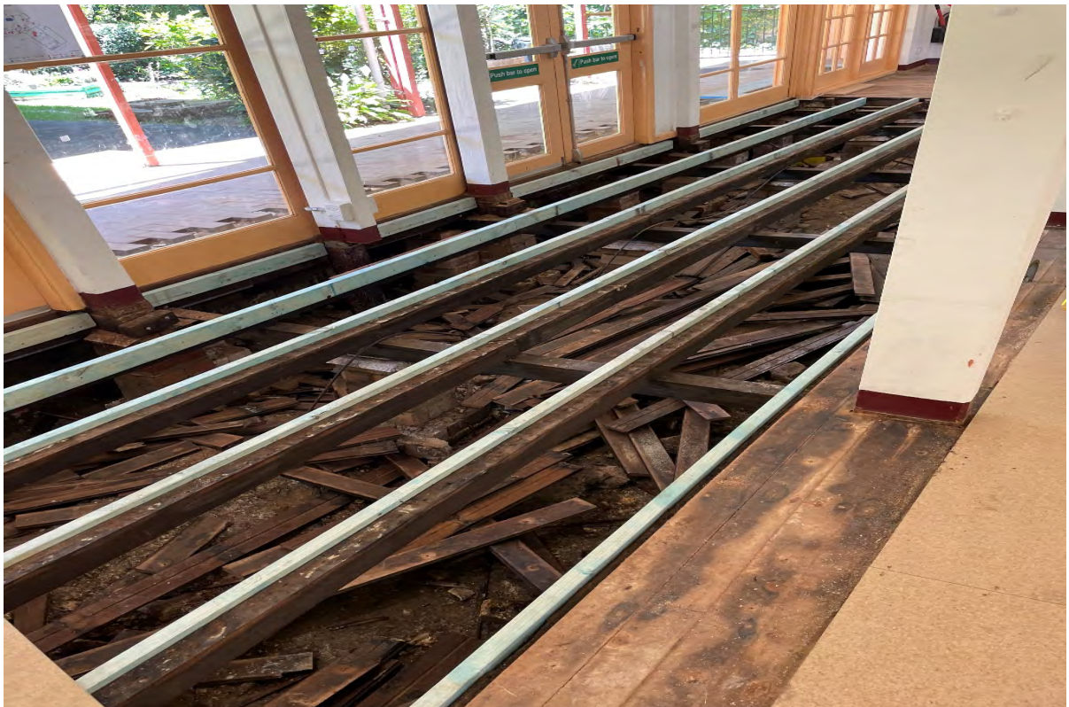
Forsyth Park Community Centre rotten flooring timbers
