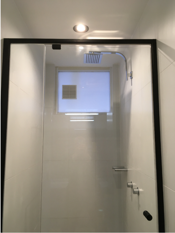
Ward Street Car Park – new shower
