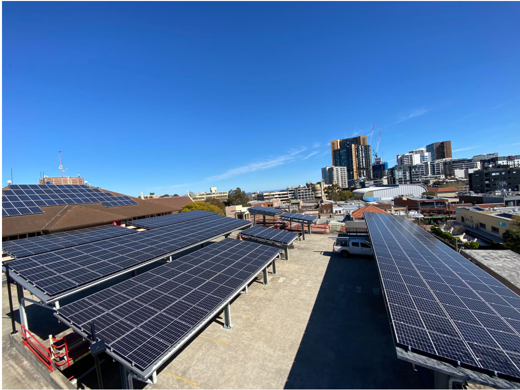
Photo 3. Holtermann Street Car Park Solar PV car ports
