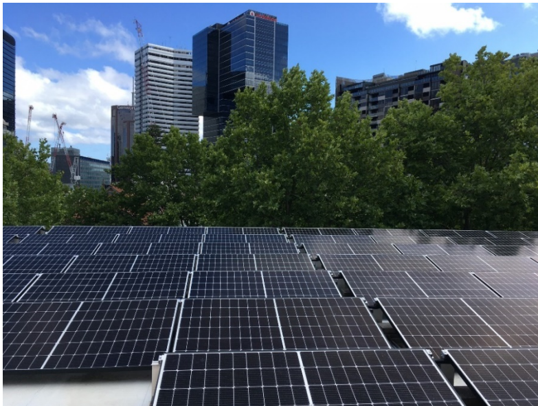
Photo 1. Council Chambers Wyllie Wing Solar PV panels
