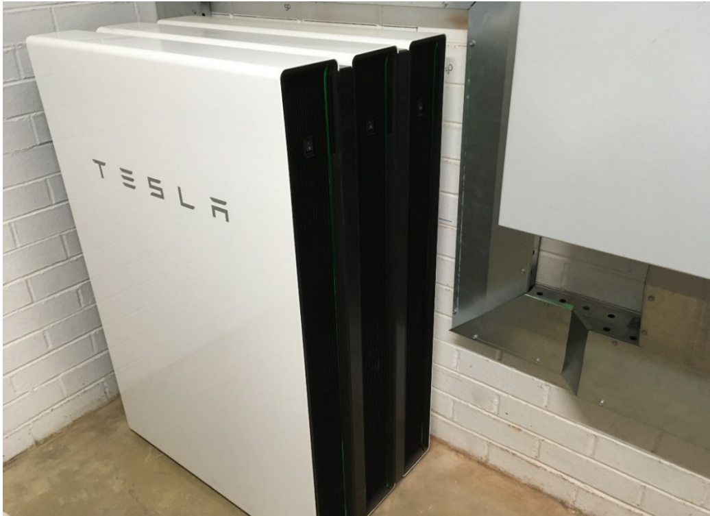
Photo 4. Tesla Batteries in Holtermann Street Car Park solar PV system
