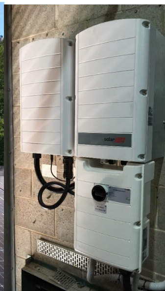
Photo 2. Council Chambers SolarEdge Inverters
