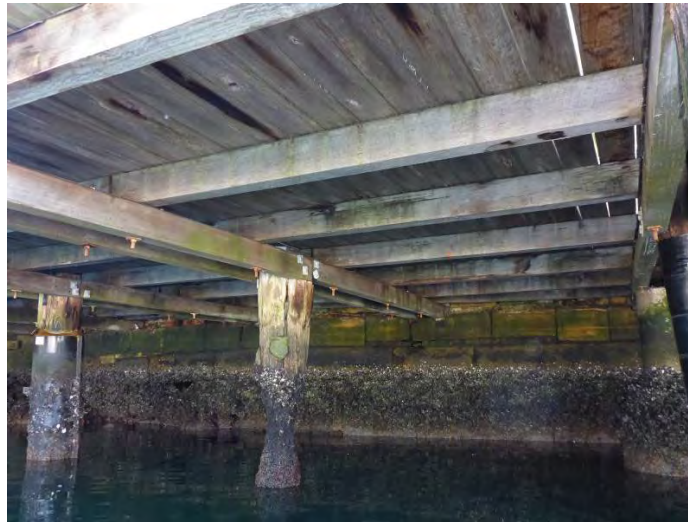
Examples failing timber piles – Wondakiah wharf
