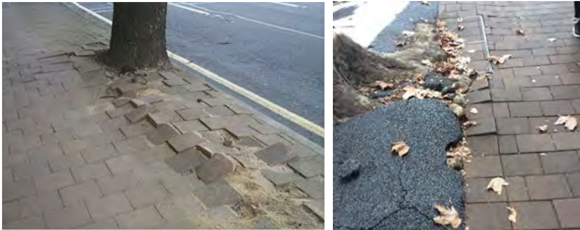
Tree root affected pavers and tree site infill
