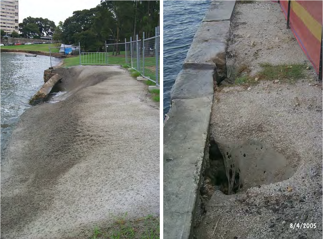
Examples of failed and failing seawalls in the North Sydney LGA – McMahons Point
