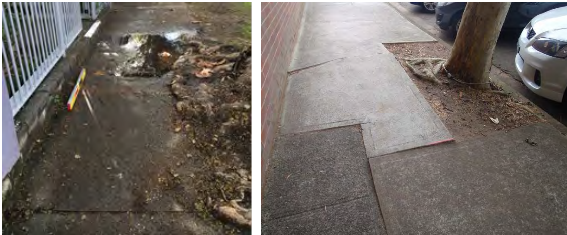
Tree root affected concrete footpath including ponding
