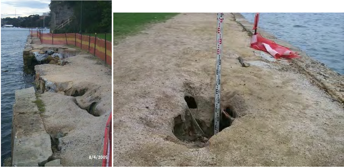
Examples of failed and failing seawalls in the North Sydney LGA – Blues Point
