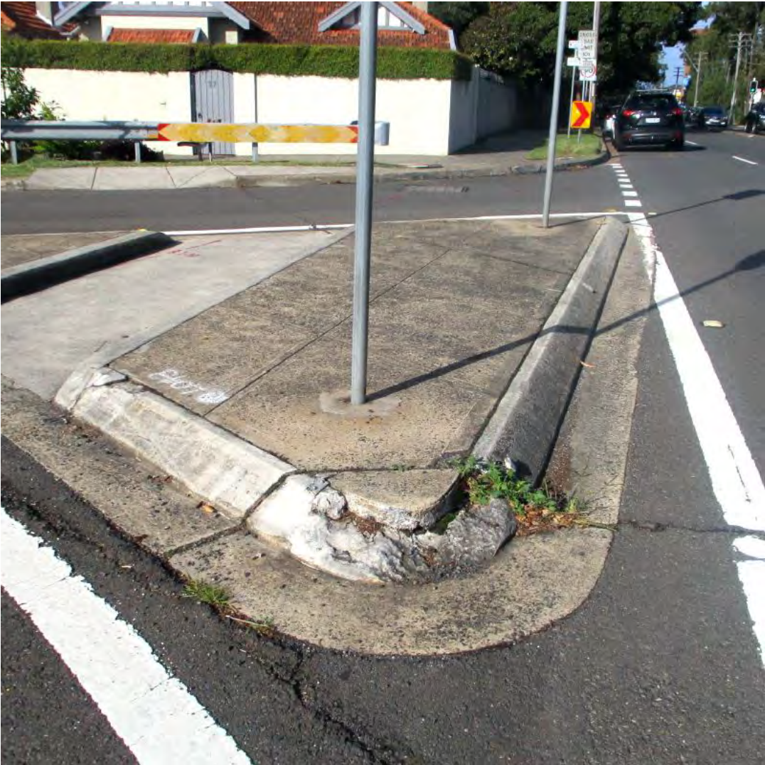
Examples of failed Traffic Facilities in the North Sydney LGA
