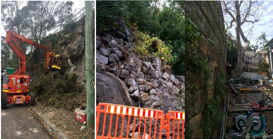
Examples of failed and failing retaining walls in the North Sydney LGA
