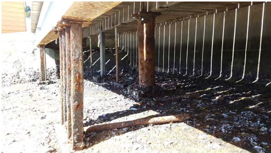
Examples failing steel piles – Boatbuilders Walk Bridge
