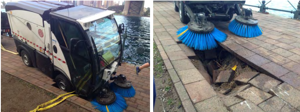
Examples of failed and failing seawalls in the North Sydney LGA – Bradfield Park
