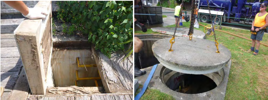
Lids are too heavy - The wood is starting to chip; they should be replaced. Lifting points rusted or broken off
