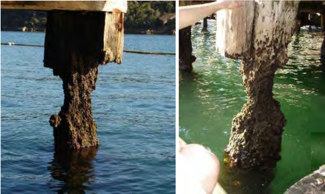
Examples of piles in very poor condition
