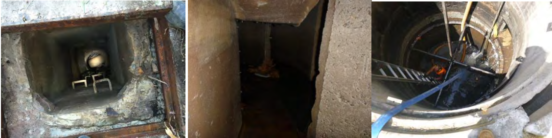
Difficult access to a lot of pits
