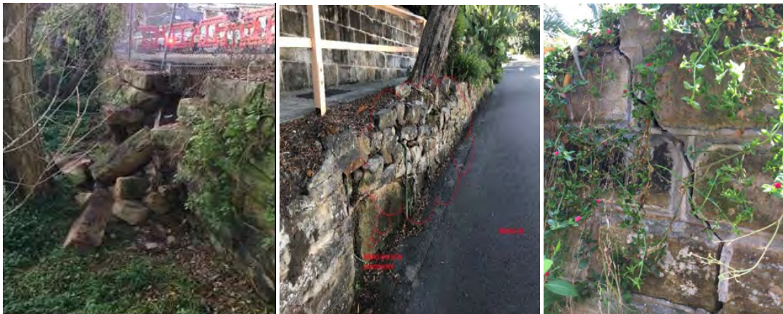
Examples of failed and failing retaining walls in the North Sydney LGA
