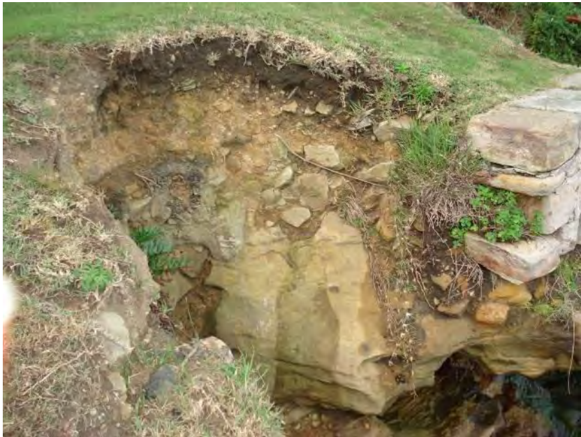
Examples of failed and failing seawalls in the North Sydney LGA – Cremorne Point
