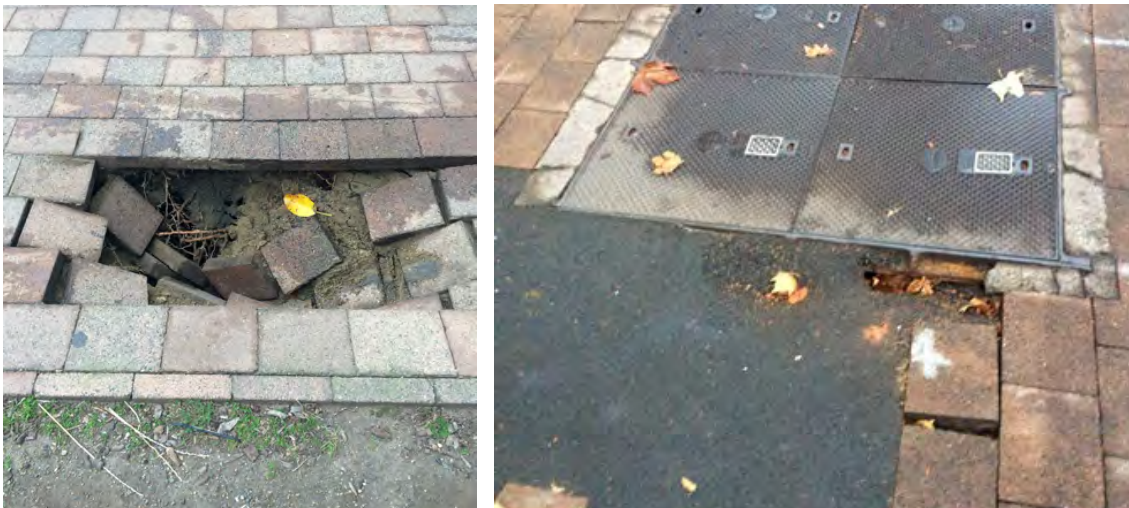
Footpath collapse due to base course wash out
