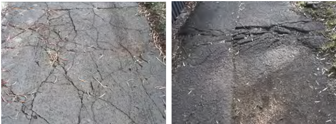
Asphaltic concrete footpath in poor condition
