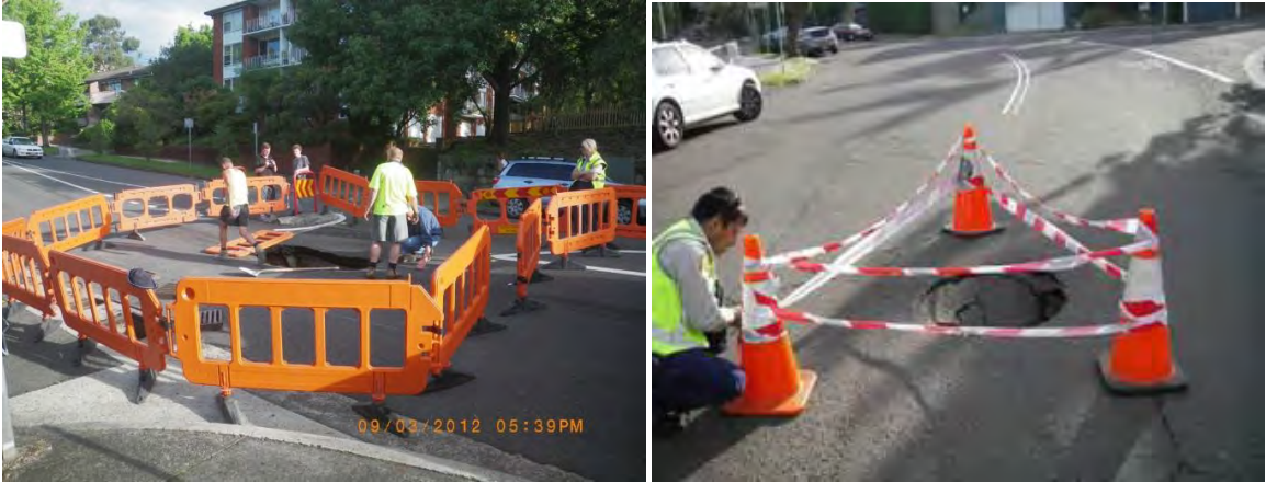
Sinkholes created from collapsed pipes and washout from leaking pipes
