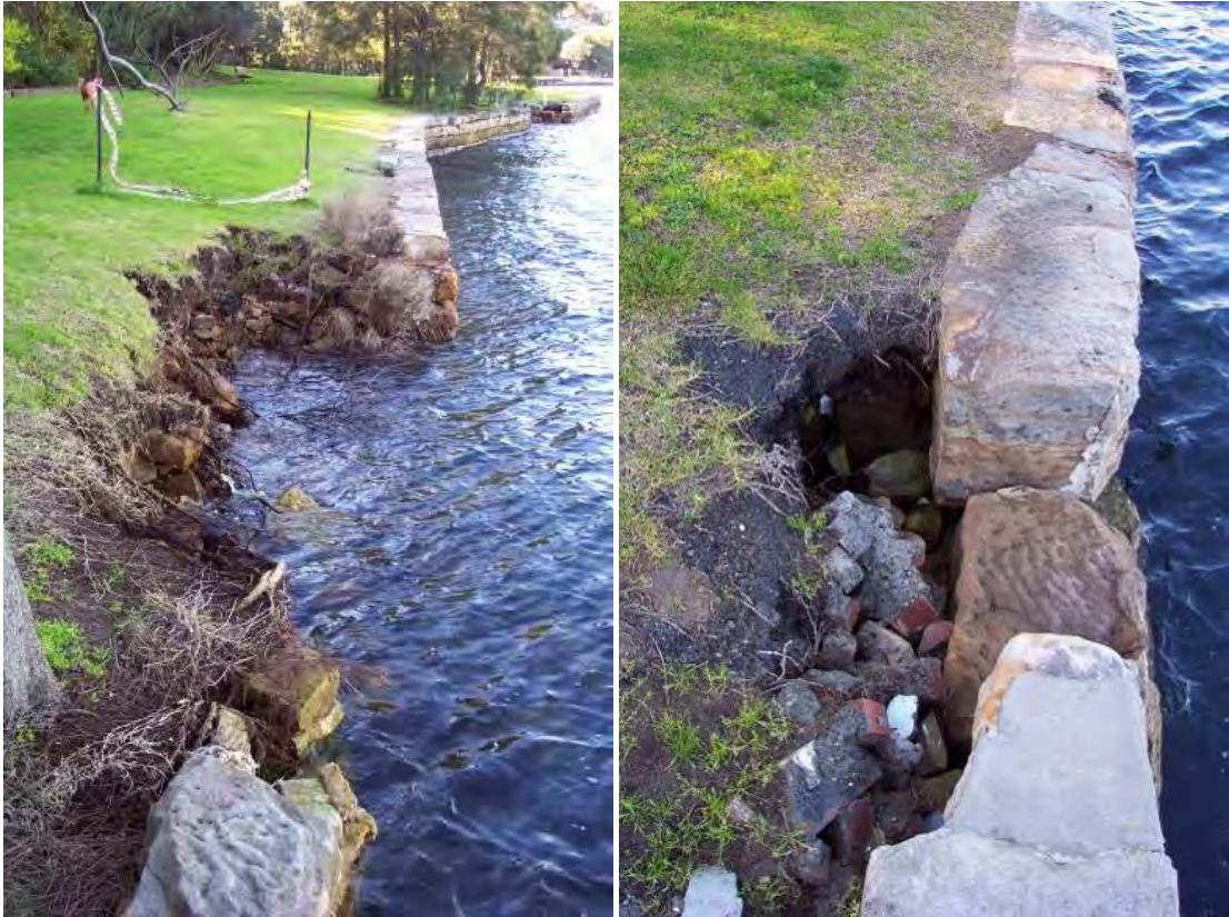
Examples of failed and failing seawalls in the North Sydney LGA – Sawmillers Reserve
