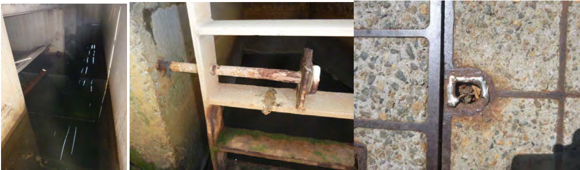
Trashracks is bent over and there is a lot of rust. Exclusion bars are rusting – lifting points are rusting due to the corrosive environment
