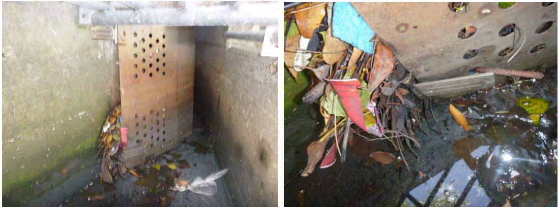
The floatables flap was jammed open due to a broken hinge and pollution trapped in it stopping it closing.
