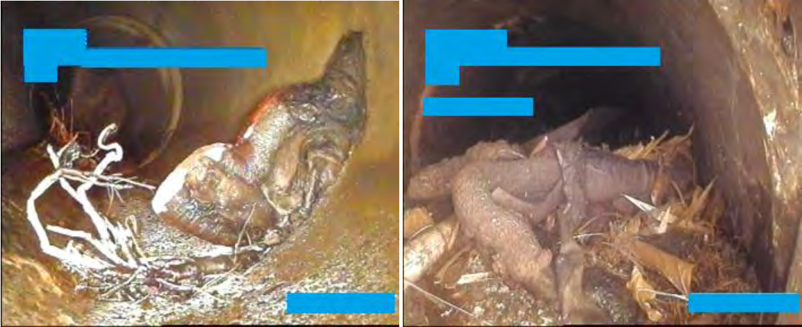
Stormwater Pipes in very poor condition – Tree root infiltrations and blocked
