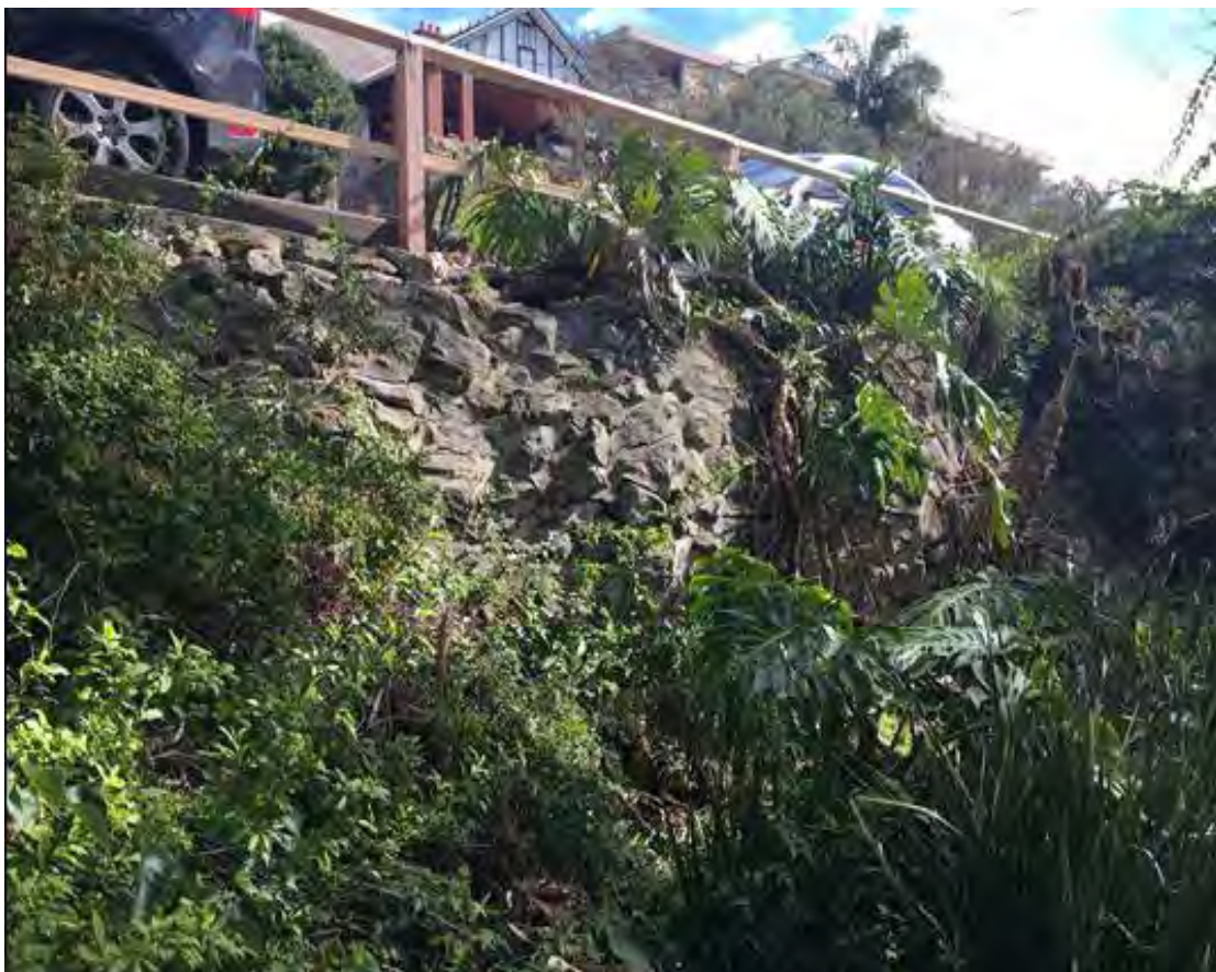
Examples of failed and failing retaining walls in the North Sydney LGA
