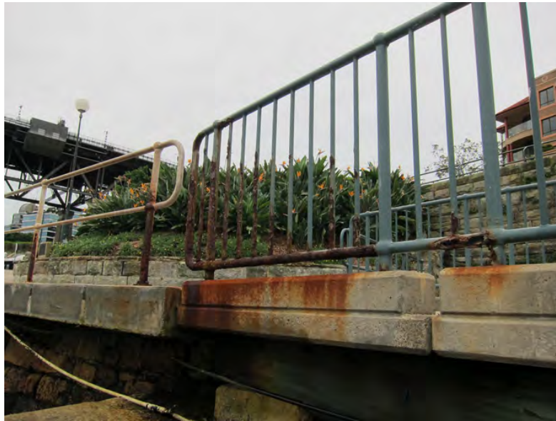
Examples corroding fence – Jefferys Street Bridge
